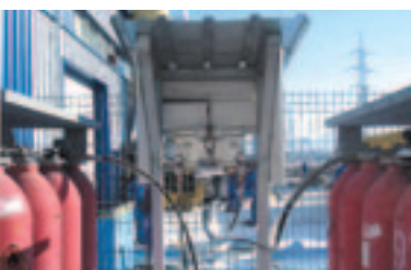
Messer Romania Gaz is setting new standards at Stabilus with a cryogenic high pressure pump.
