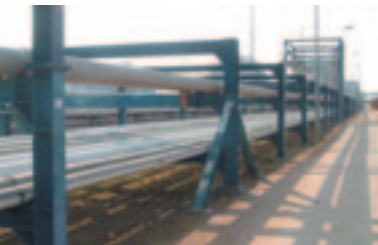
Messer Carburos operates a pipeline system to supply its industrial customers.
