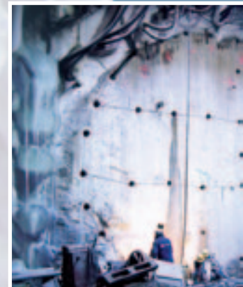
For the extension of the Vienna subway network, the ground was frozen with nitrogen from Messer in order to prevent subsidence (see also page 26).
