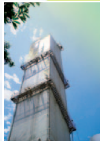
In mid-June 2005, XMG commissioned a new air separation plant in Hunan, China. It has a daily capacity of 550 tons (see also page 60).
