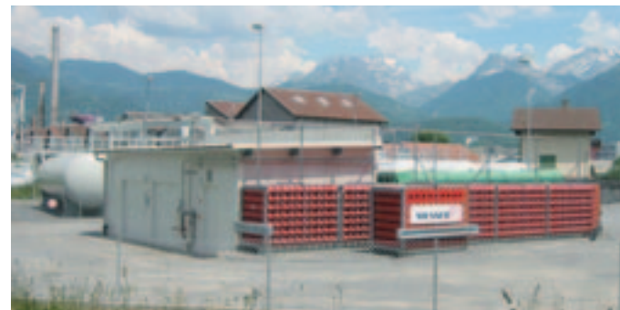
Compressor station for hydrogen with storage facility in Monthey.
