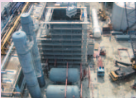
Messer has built a new air separation plant in Smederevo, Serbia, which went into service at the beginning of 2006.
